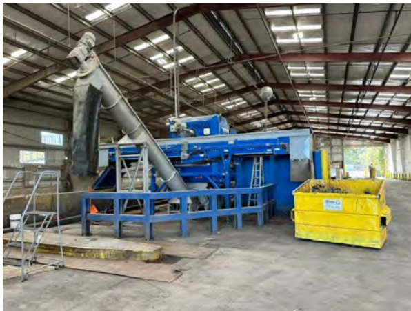
Figure 4-1. Commercial Food Waste Depackaging System at MSS
