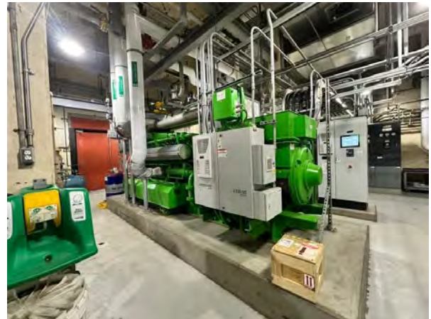
Figure 4-4. Jenbacher Internal Combustion Engine-Generator Set
