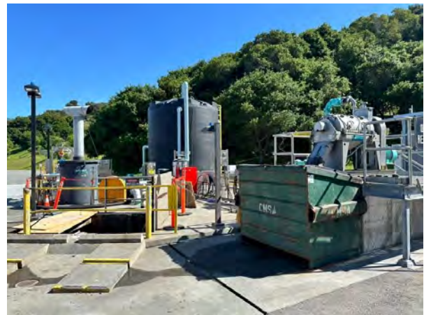
Figure 4-2. Food Waste Slurry Receiving/Processing System at CMSA
