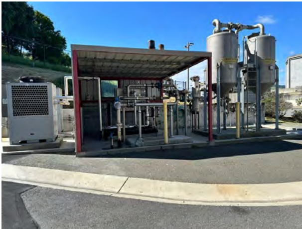
Figure 4-3. Biogas Cleanup System at CMSA
